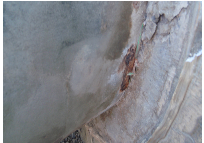
A corrosion patch found at the interface location.
